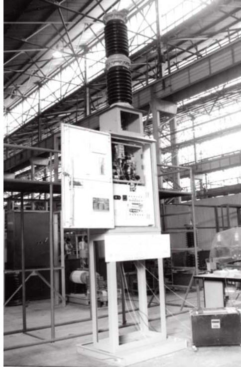
Fig. 3.14: 25 kV outdoor track-side vacuum switchgear
